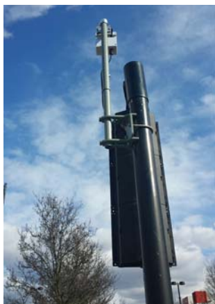
Access point used as part of SCOOT installation
