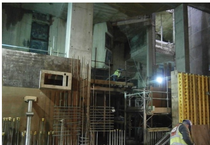
Fixing and pouring walls in the LU station box at Bank station
